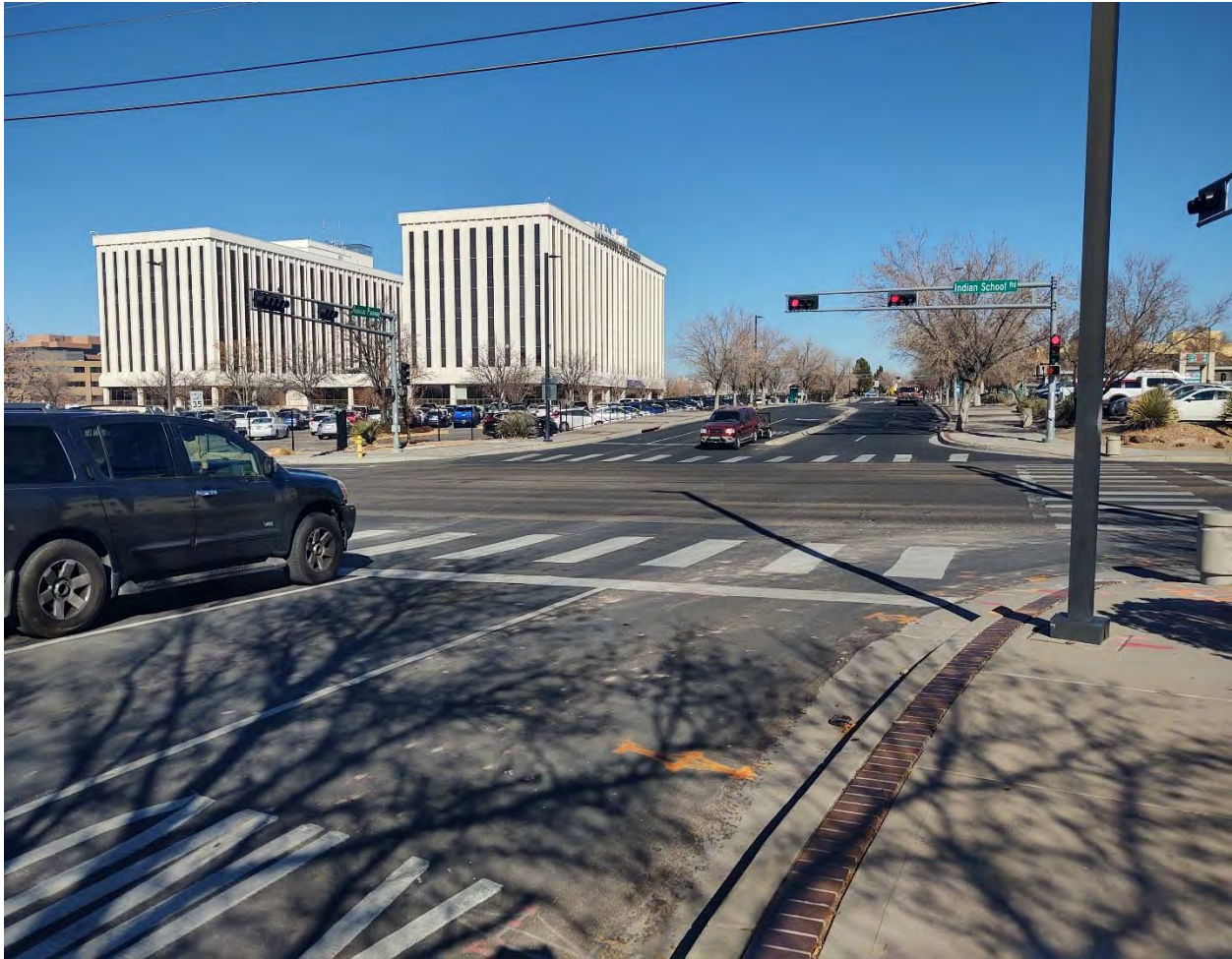
Photo 1: Indian School Road at Americas Parkway - Looking North. Low to moderate severity of raveling, oxidation, and weathering. Low severity transverse cracking of asphalt concrete.
