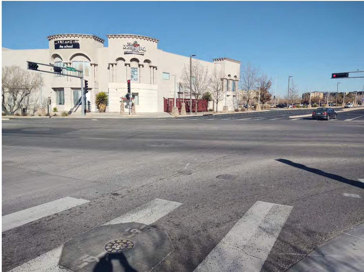
Photo 4: Indian School Road at Q Street - Looking North. Low to moderate severity raveling, oxidation, weathering, and patching. Low severity longitudinal and transverse cracking of asphalt concrete.
