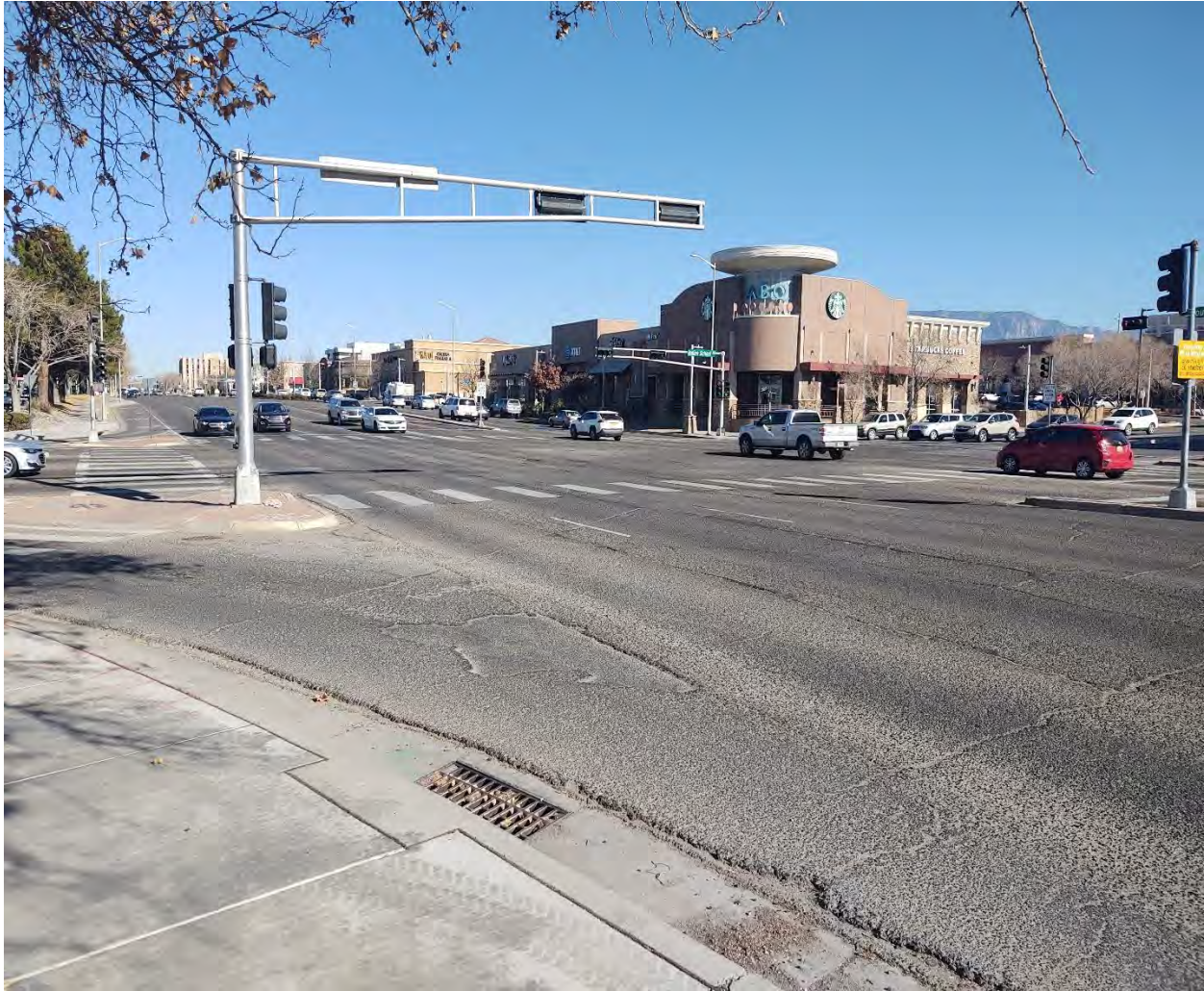
Photo 2: Indian School Road at Louisiana Boulevard - Looking North. Low to moderate severity raveling, oxidation, weathering, and lifting/stripping of overlay/OGFC. Low to moderate severity longitudinal and transverse cracking of asphalt concrete.
