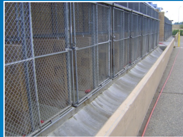
Collection of pet stall wash water for disposal to sanitary sewer.
