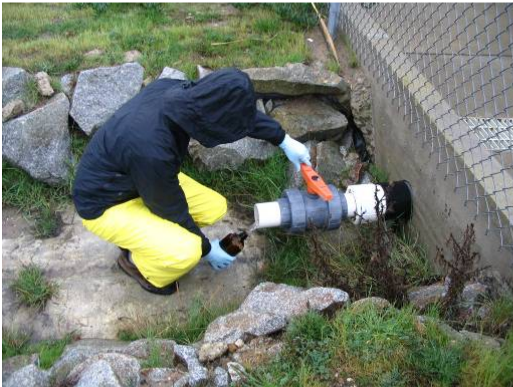
Stormwater discharges to the slot drain and is conveyed offsite through a valved pipe.
