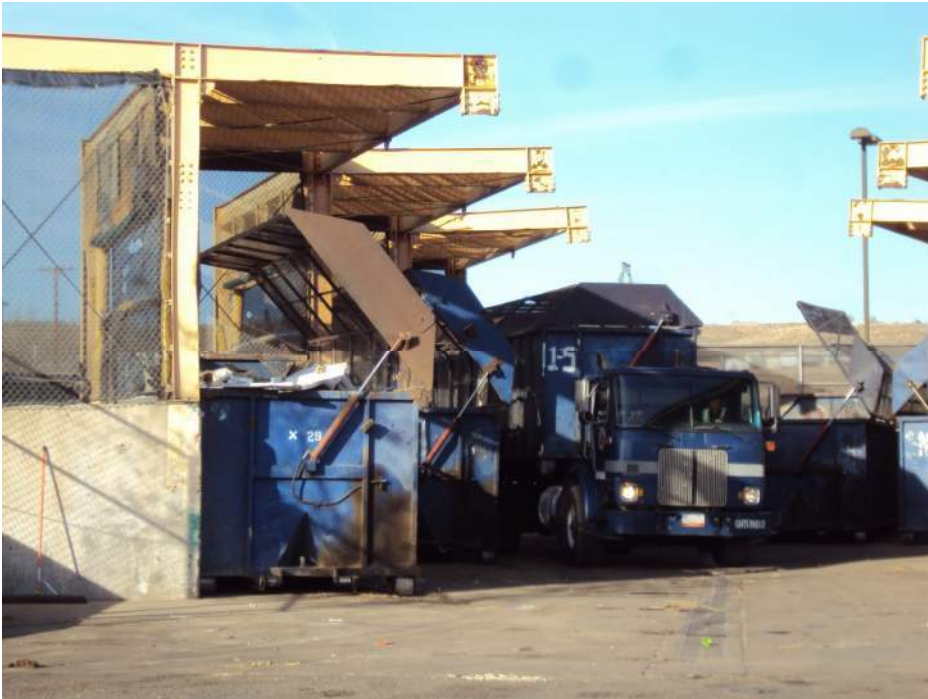
IMG_130: Collection, maintenance, and mobile fueling area with trench drain
