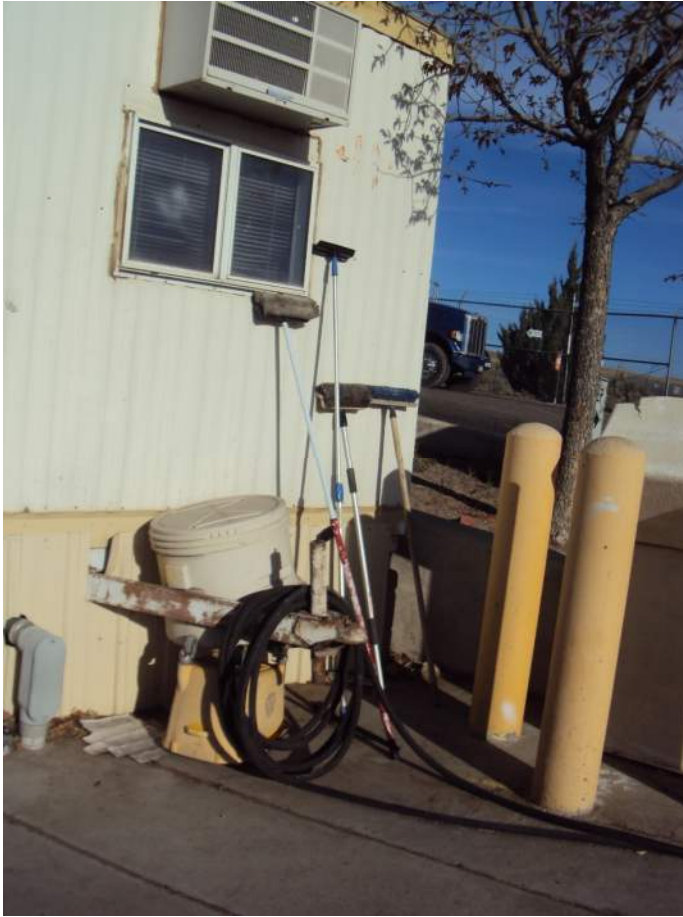
IMG_144: Hose bib and hose for equipment wash down
