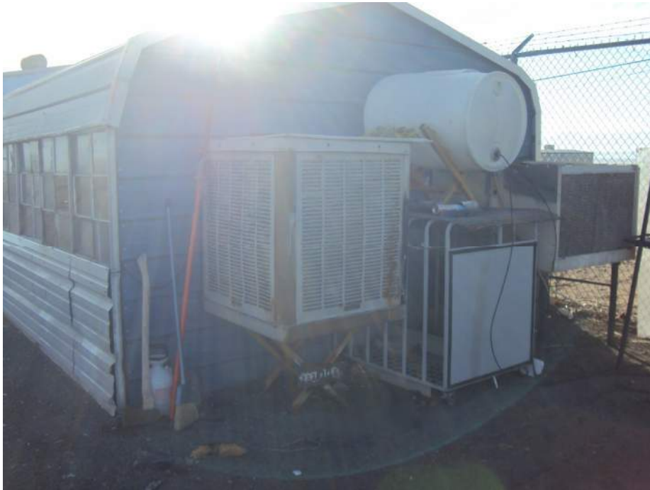
IMG_111: Building HVAC equipment includes a water barrel
