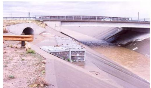
Alameda Debris Screen and North Diversion Channel (4/3/04)
