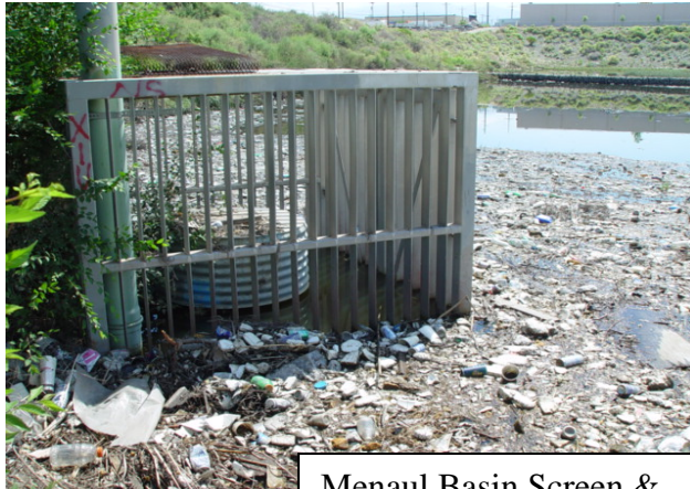
Manaul Basin Screen & Baffled Pipe Outlet
