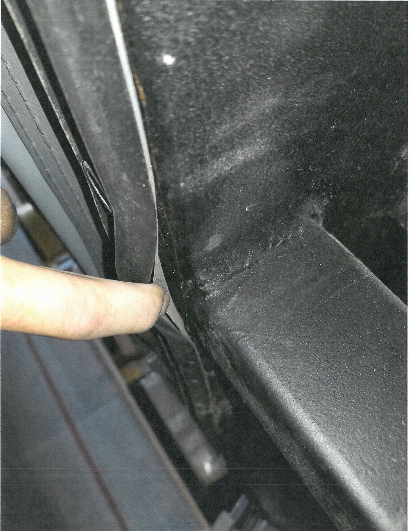
1716- Front of joint/bellows welds questionable & rusting
