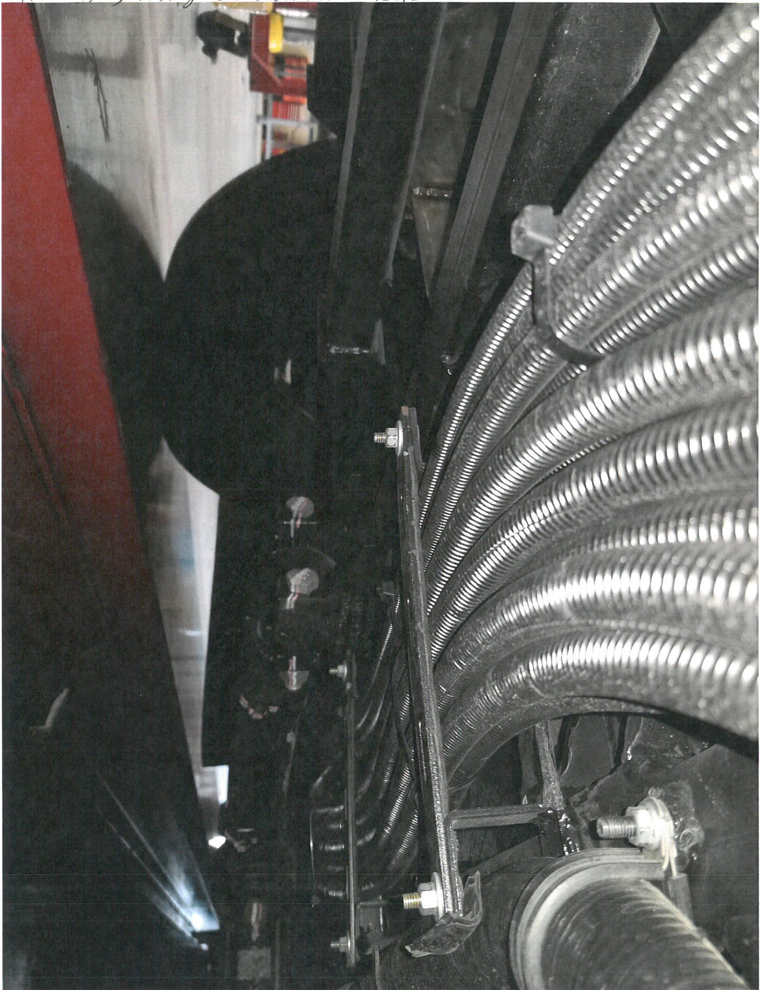
1716-Cables rubbing on Securement brackets
