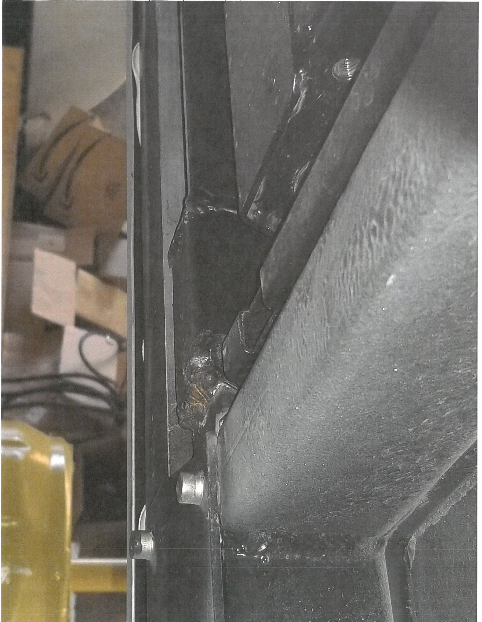
1708 poor and rusting welds, Bridge plate frame
