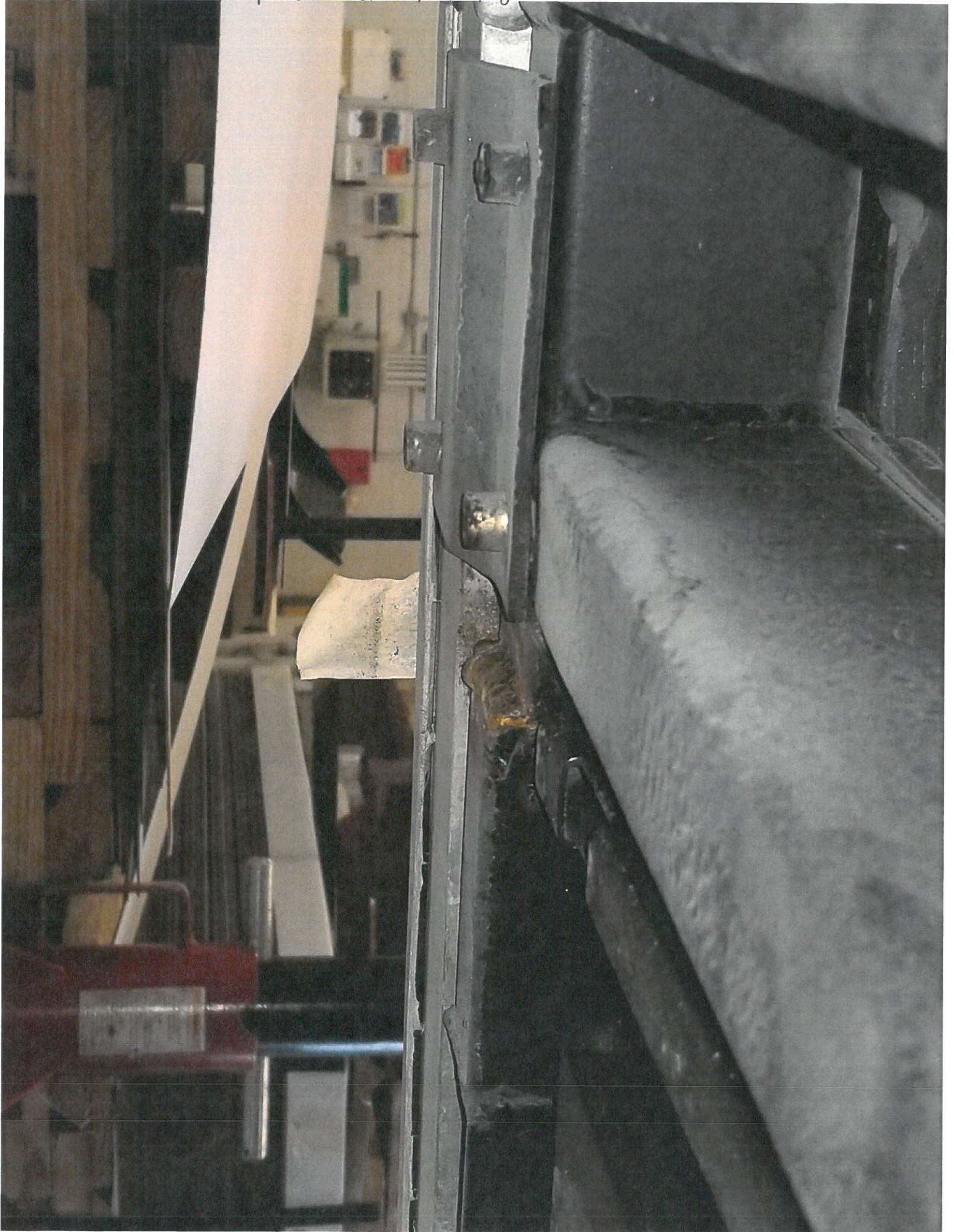
1708 CLS Bridge plate welds rusting
