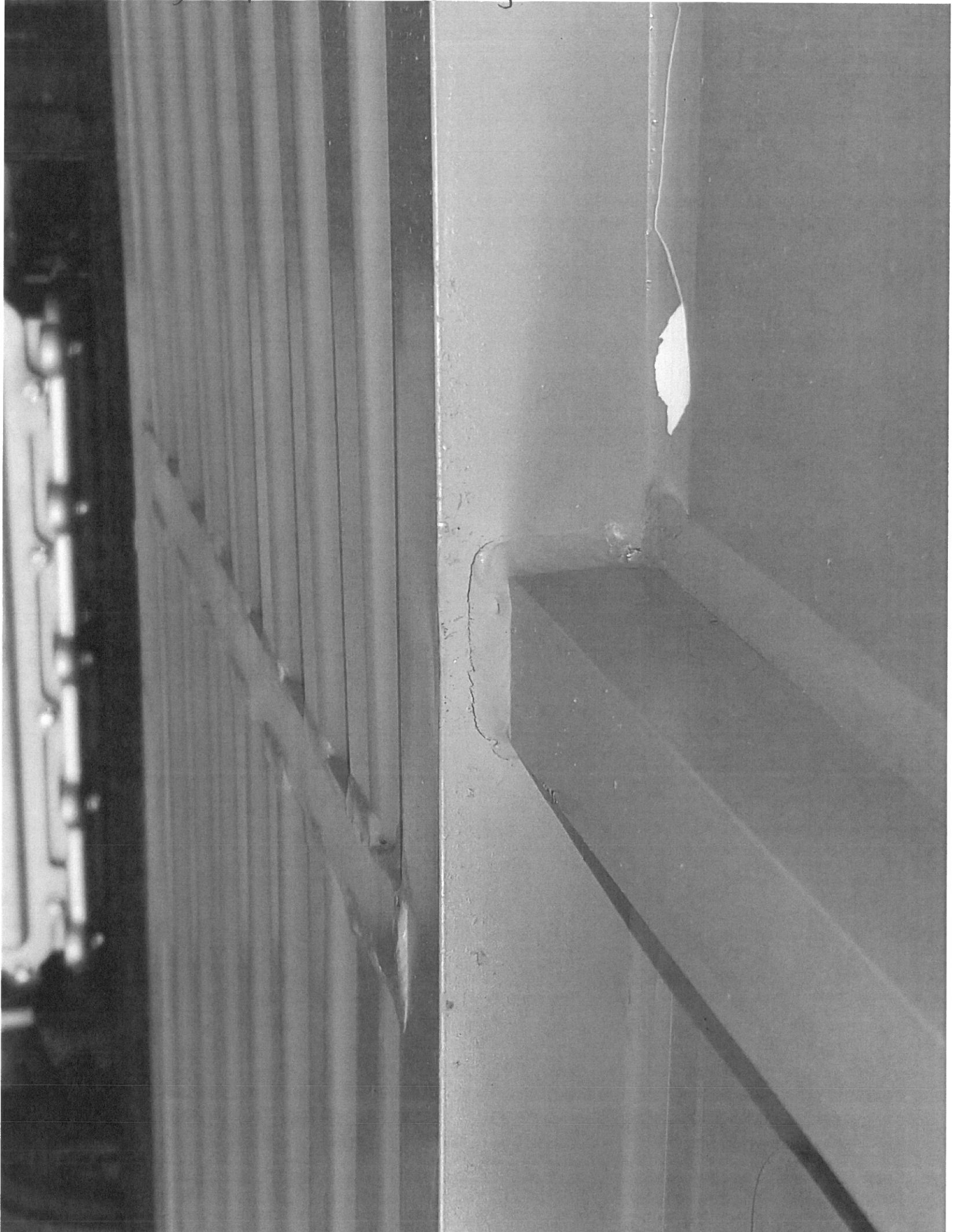
1708- Engine Cnpt Door welds cracking
