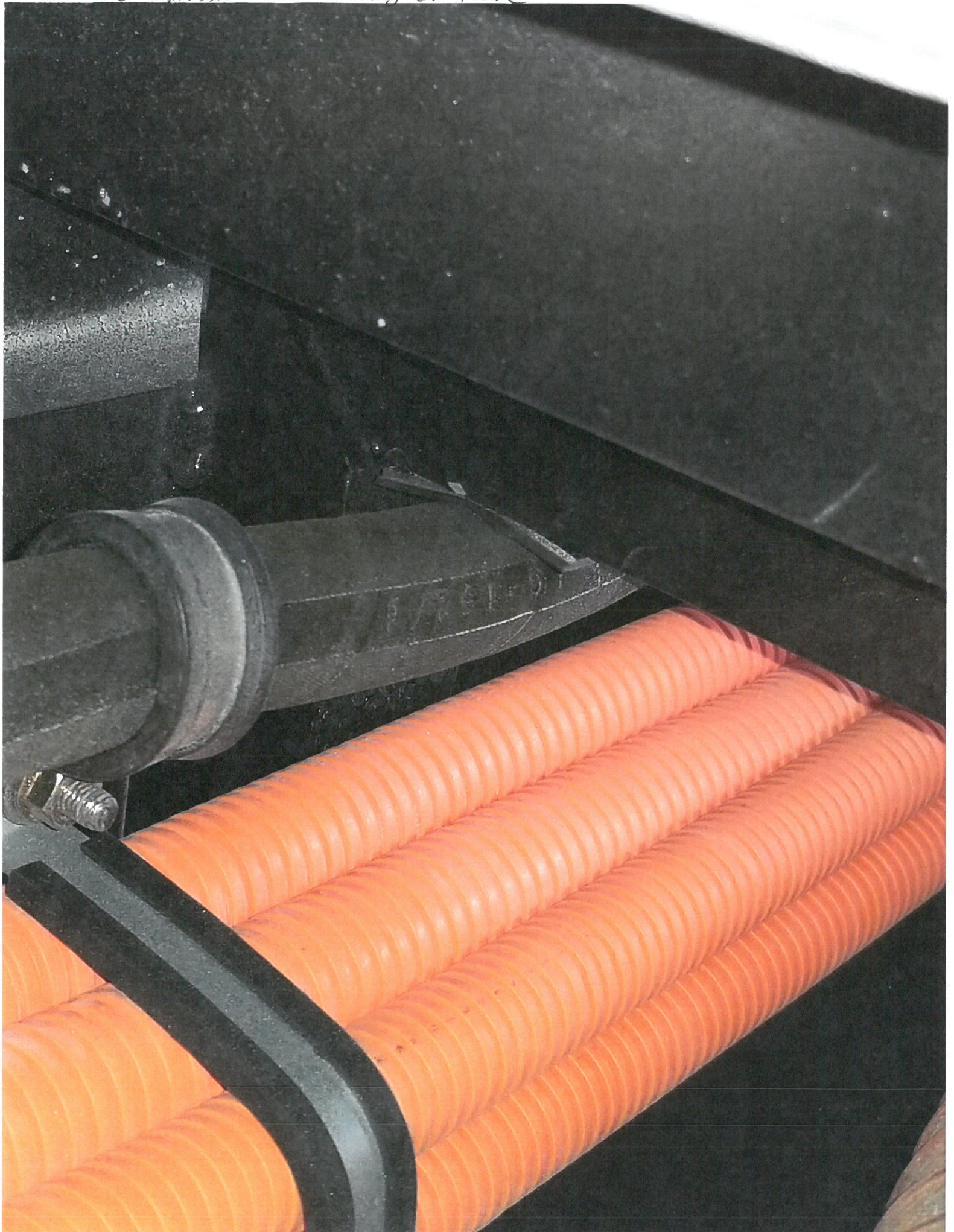
1708- Fire Suppression line rubbing on Frame
