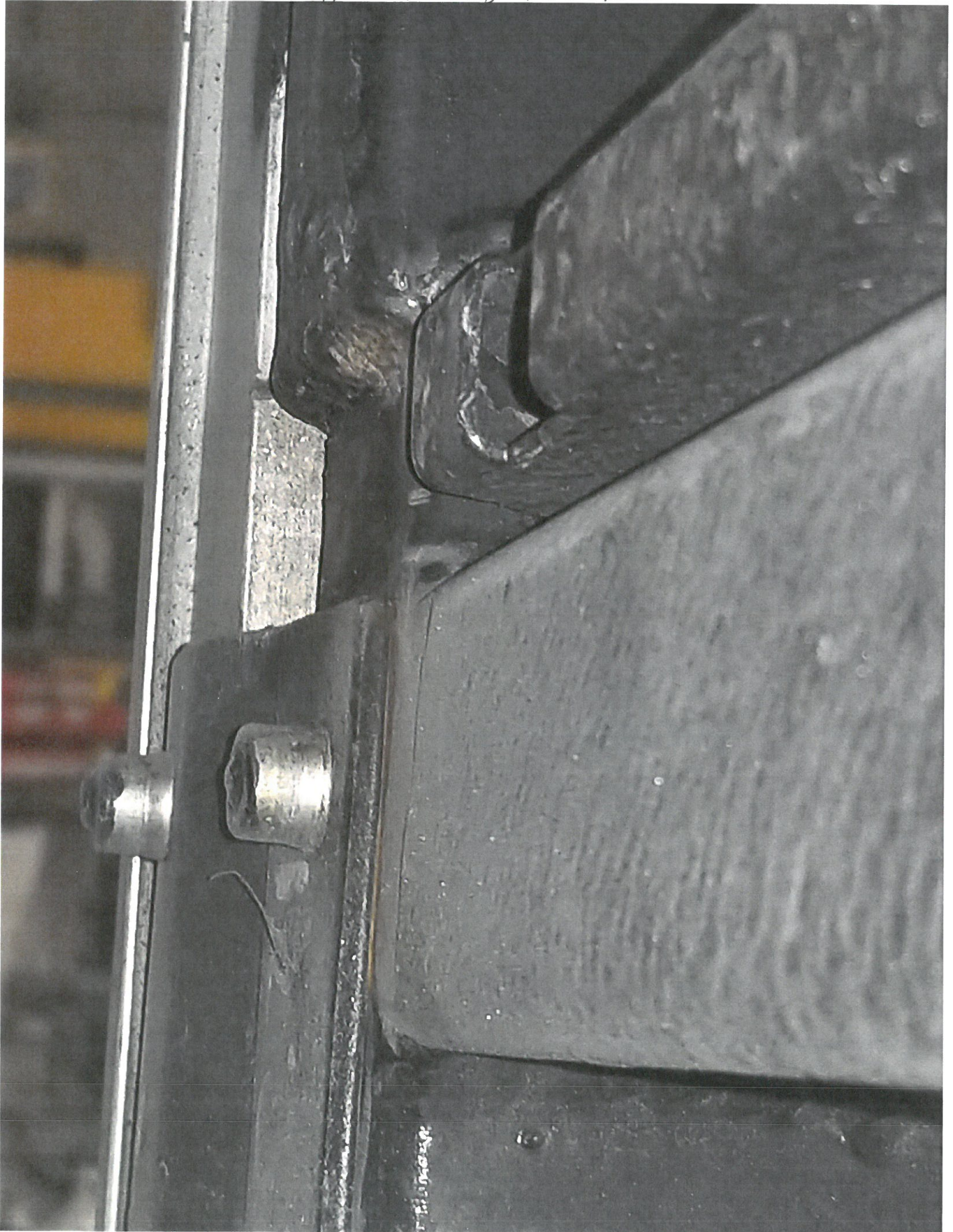
1708 poor and rusty welds. Bridge plate frame
