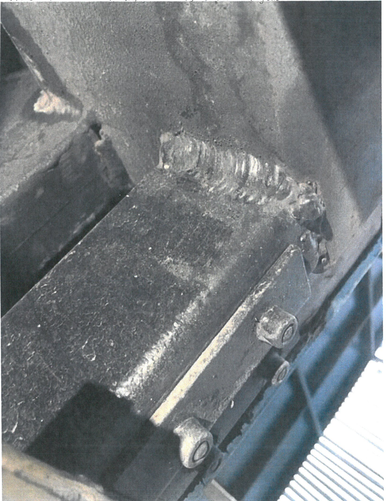
1702 Poor and incomplete welds, rear of joint
