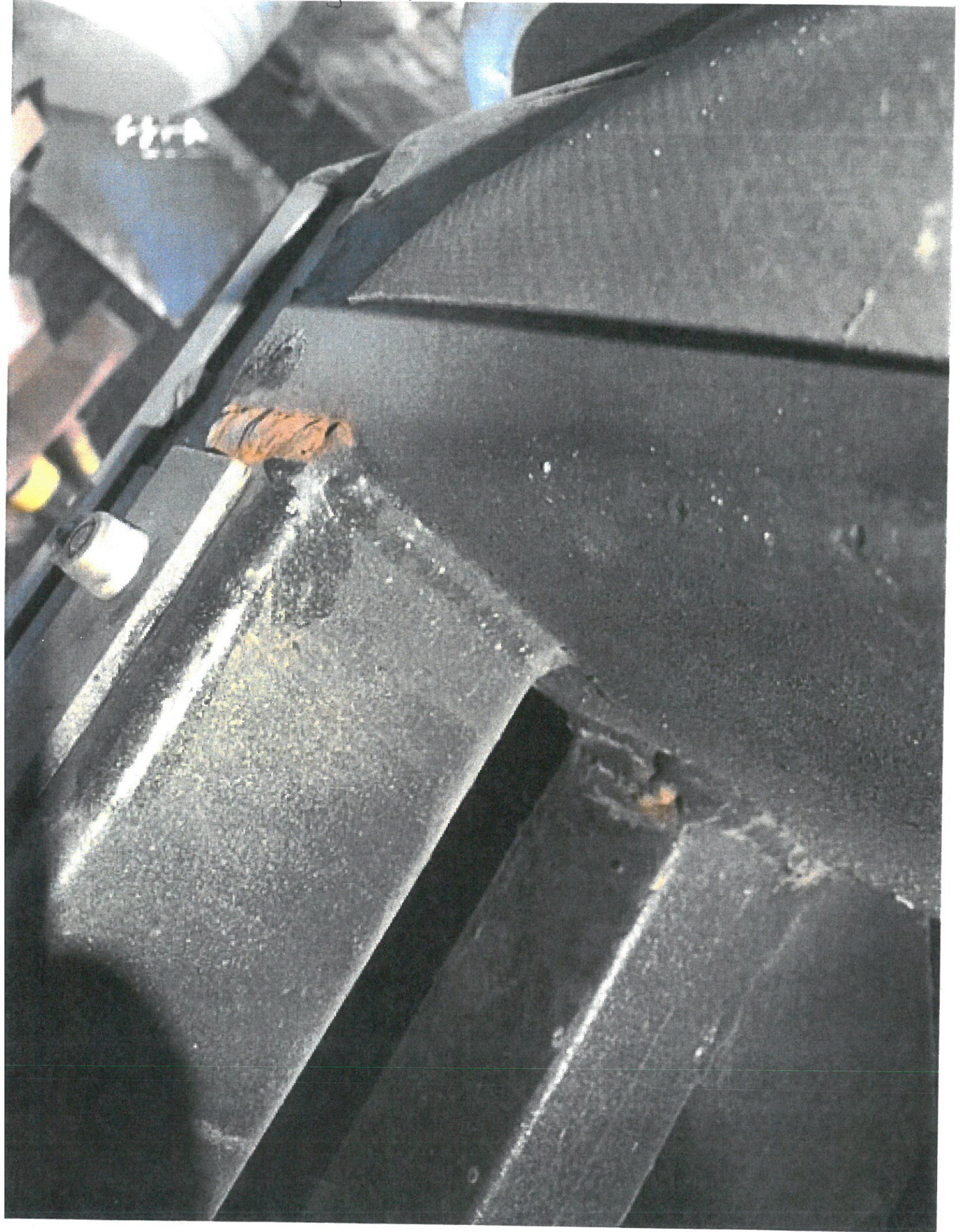
1702 Poor and rusting welds
