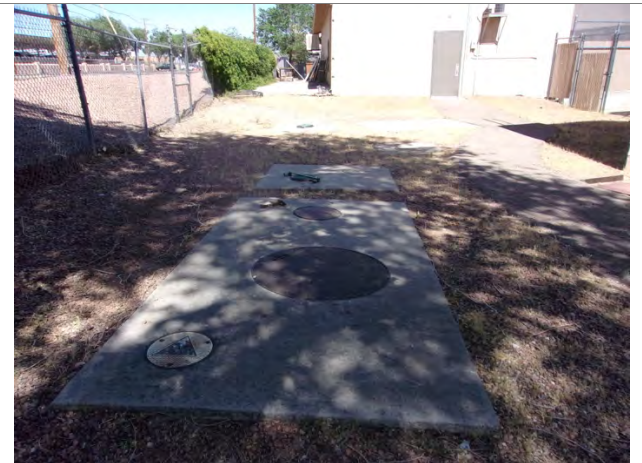
Photo 18: USTs located on the south side of the powerplant.
