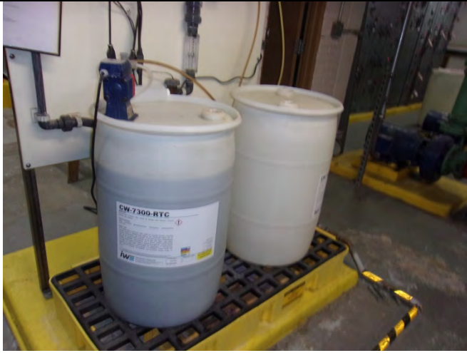
Photo 13: Water treatment compounds inside the powerplant.
