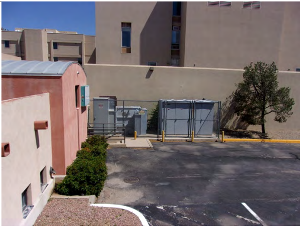
Photo 15: Electrical equipment on the south side of the main building.
