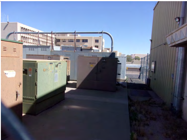
Photo 11: Transformers adjacent to the power plant.
