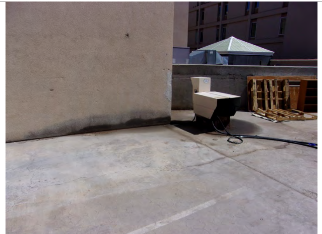
Photo 16: Hydraulic oil strain outside of the trash compactor.
