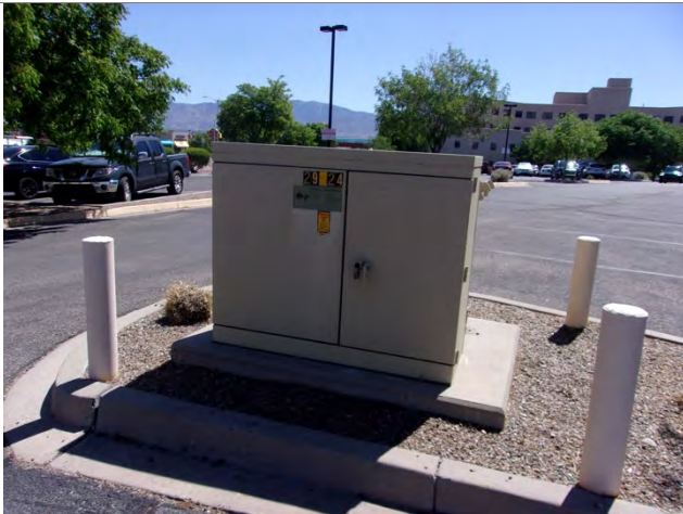
Photo 9: Transformer in the northwest corner of the subject property. (Station No. 2924).
