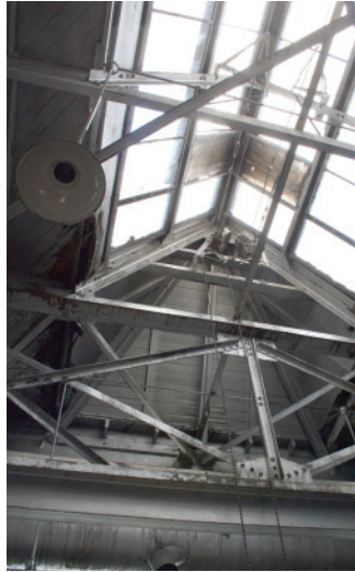
Gear/Pulley mechanism for skylight operation.
