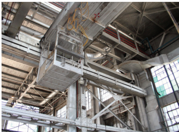
Crane operator workstation, Bay #2.
