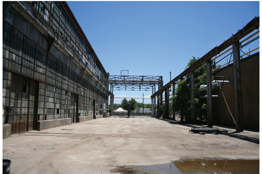
Bridge Crane, View from West Elevation.
