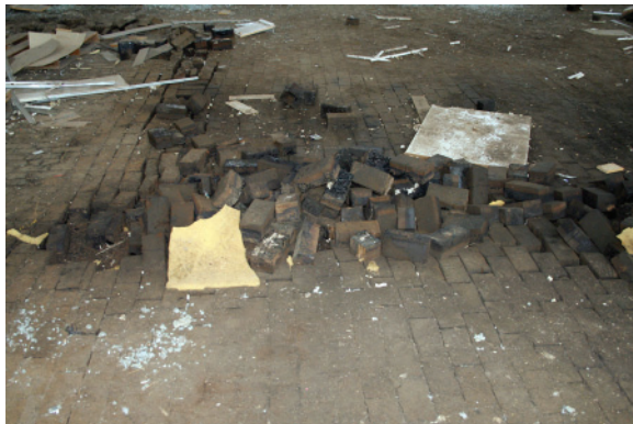
Damaged flooring, 3" thick creosoted end-grain wood blocks
