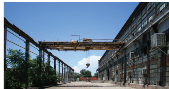
South bay, Exterior loading crane.
