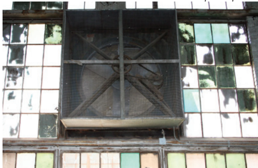
Fan equipment at Glazed Elevation.
