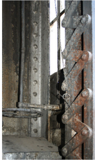
Crank mechanism for skylight operation.
