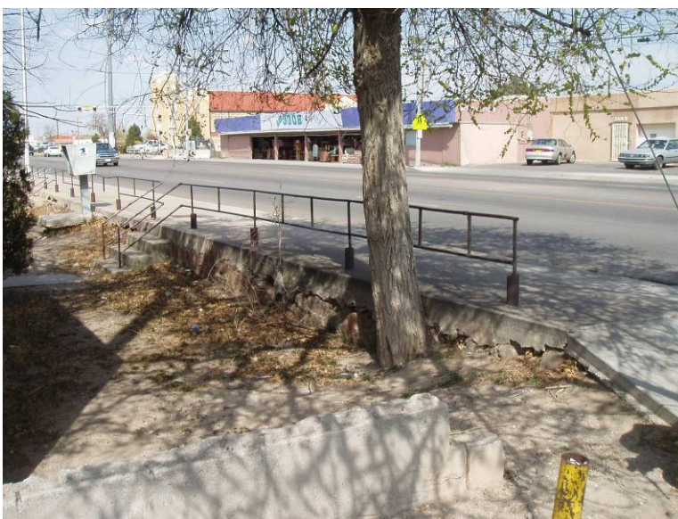
The sidewalk is not ADA compliant and the foundation is crumbling.
