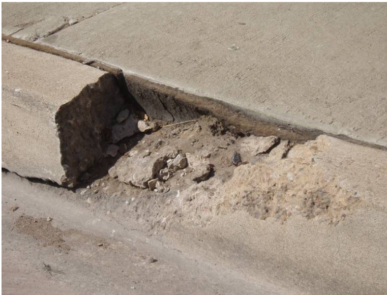
Curbs are broken and crumbling in many places along the street
