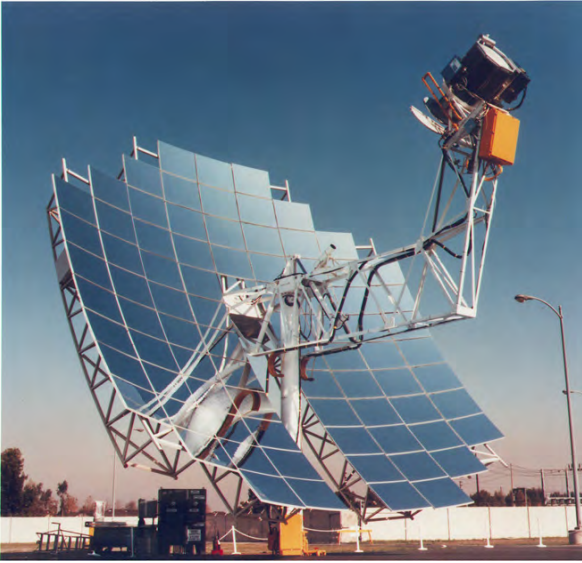
Stirling Concentrating Solar Dish/Engine Facility
