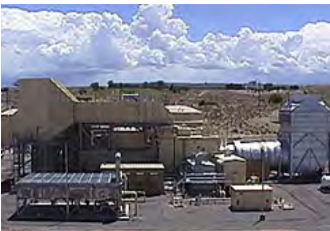
Simple-Cycle Gas Turbine Generating Station
