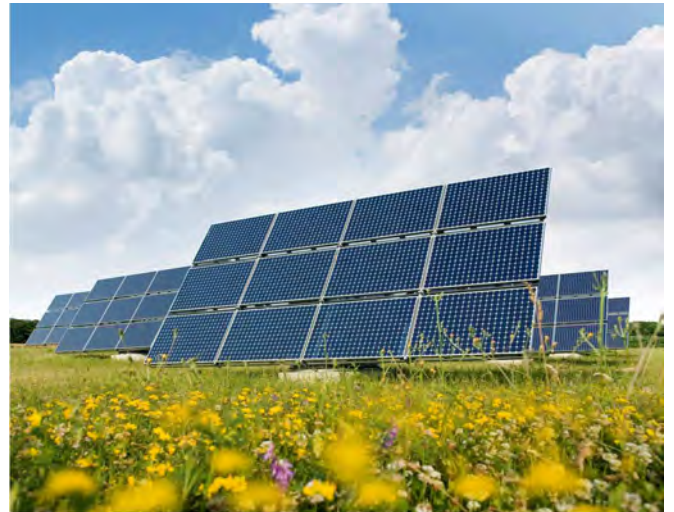
Solar Photovoltaic Ground-Mounted Installation or Utility Facility
