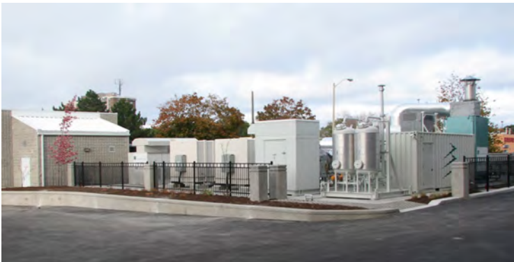
Fuel Cell Facility
