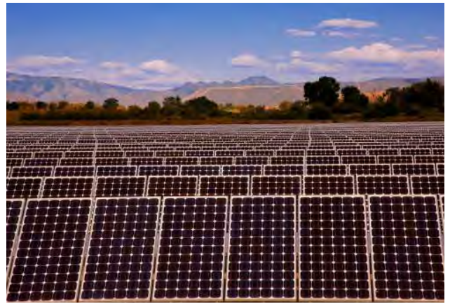
Solar Photovoltaic Yard Utility Facility
