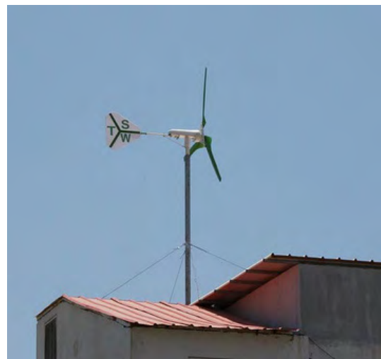
Roof-Mounted Wind Installation
