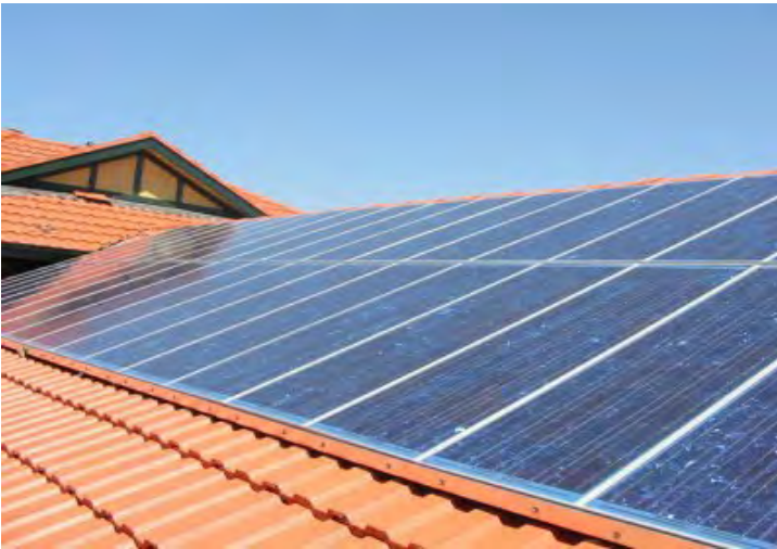
Solar Photovoltaic Roof-Mounted Installation
