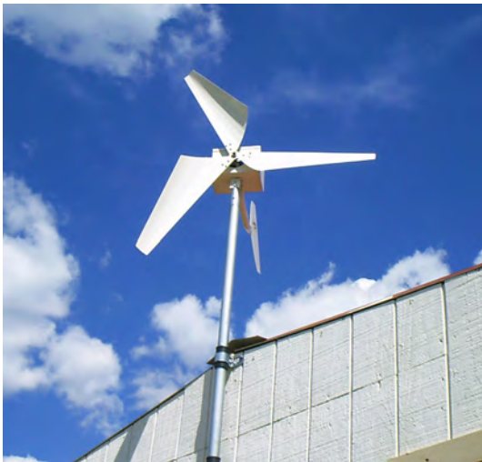
Building-Mounted Wind Installation
