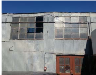
Building Exterior – Broken glass
